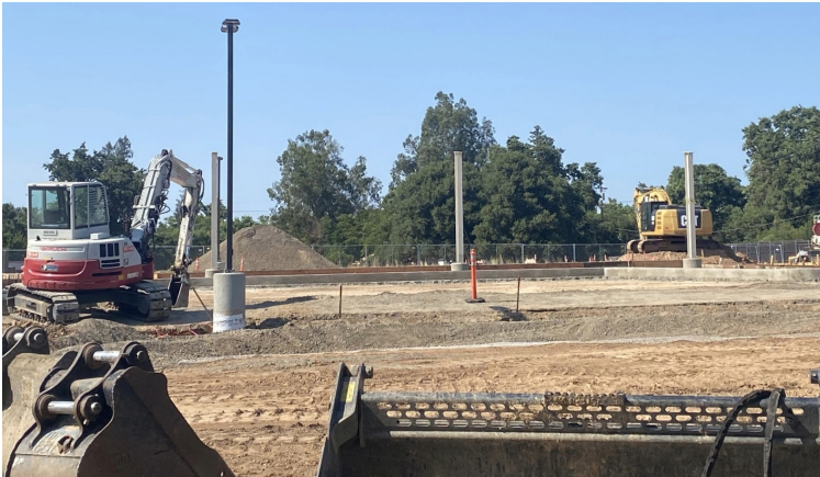
Concrete curbs and lighting have been installed as work continues on the parking lot renovation project.
